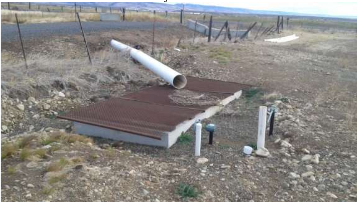
Below: The control structure which draws water from the main irrigation ditch for the site.
